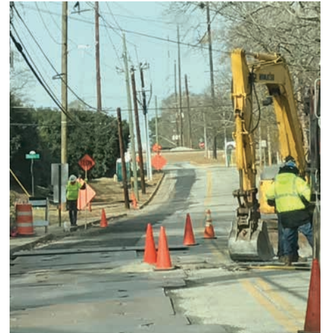
Entering the final phase of the Clarkston Streetscape Water Main Relocation Project, traffic detours and control will continue to impact drivers in Clarkston.
