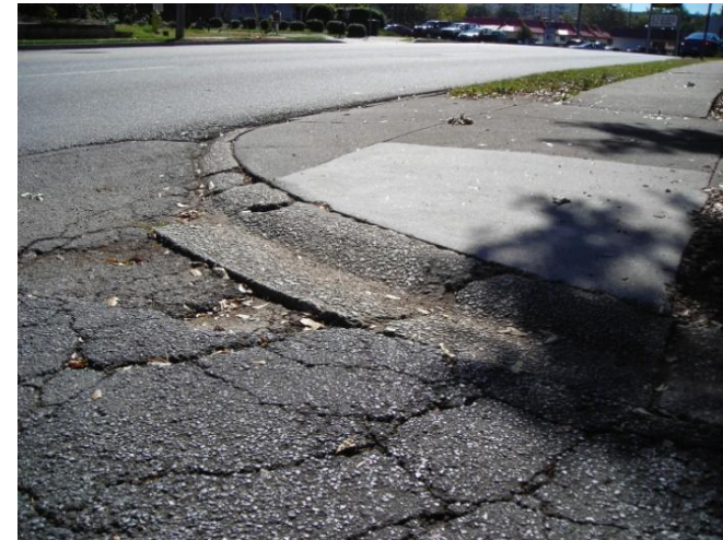
Patchy sidewalks and poorly maintained curb ramps make it difficult for those in wheelchairs to safely navigate the built environment
