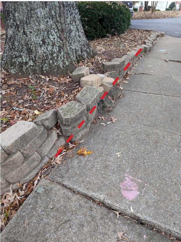
Pic 1: Location of root flare overgrowth. Shear cut here.
